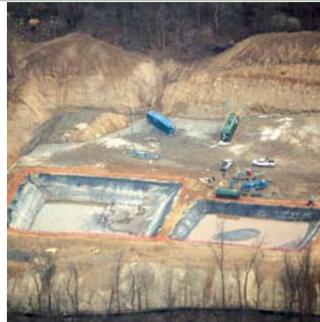
▲ Wastewater is often stored in open-air treatment ponds, like these in Washington County, which can leak or overflow.
