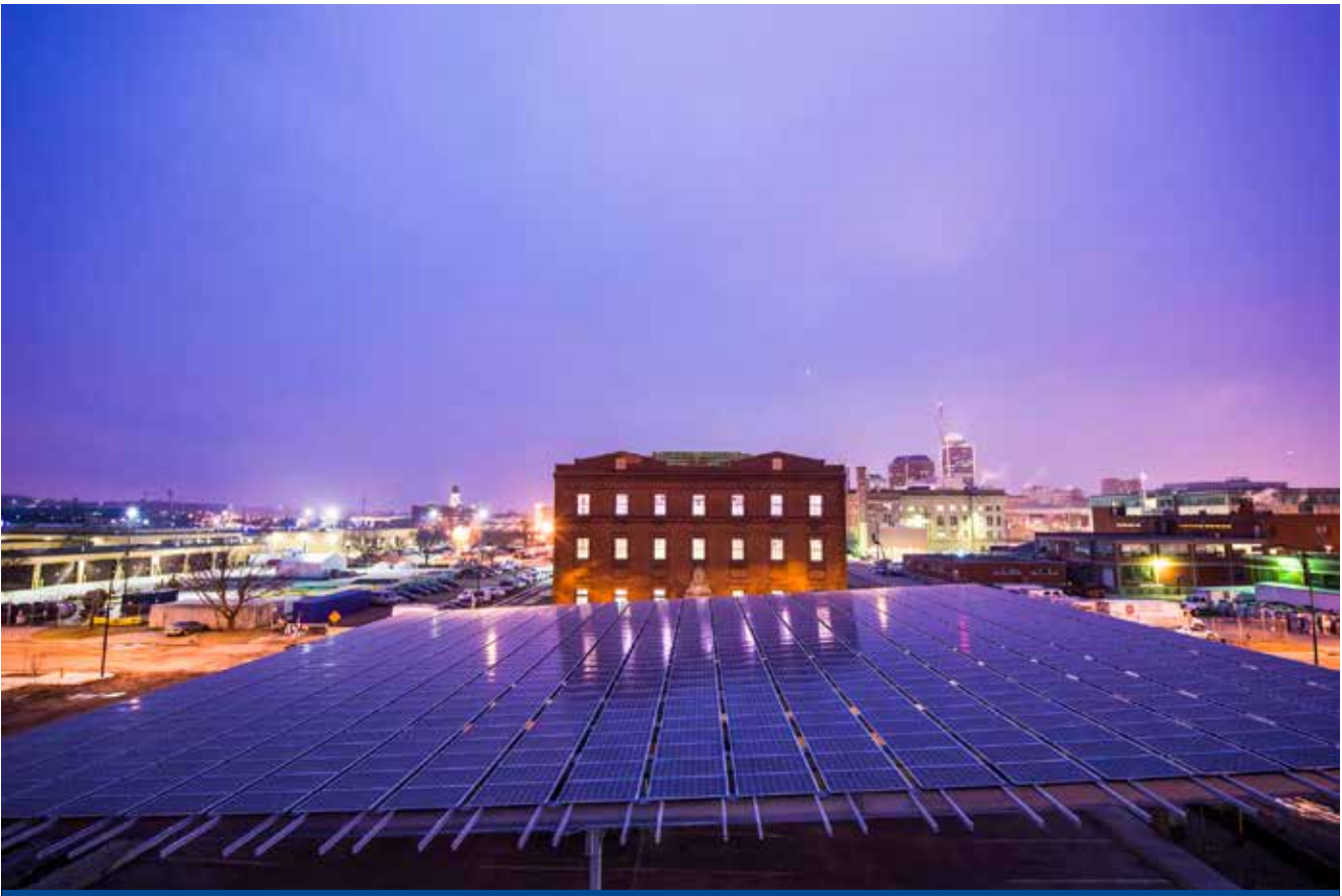
Solar panels generate power at the Market One commercial building in Des Moines, Iowa.
